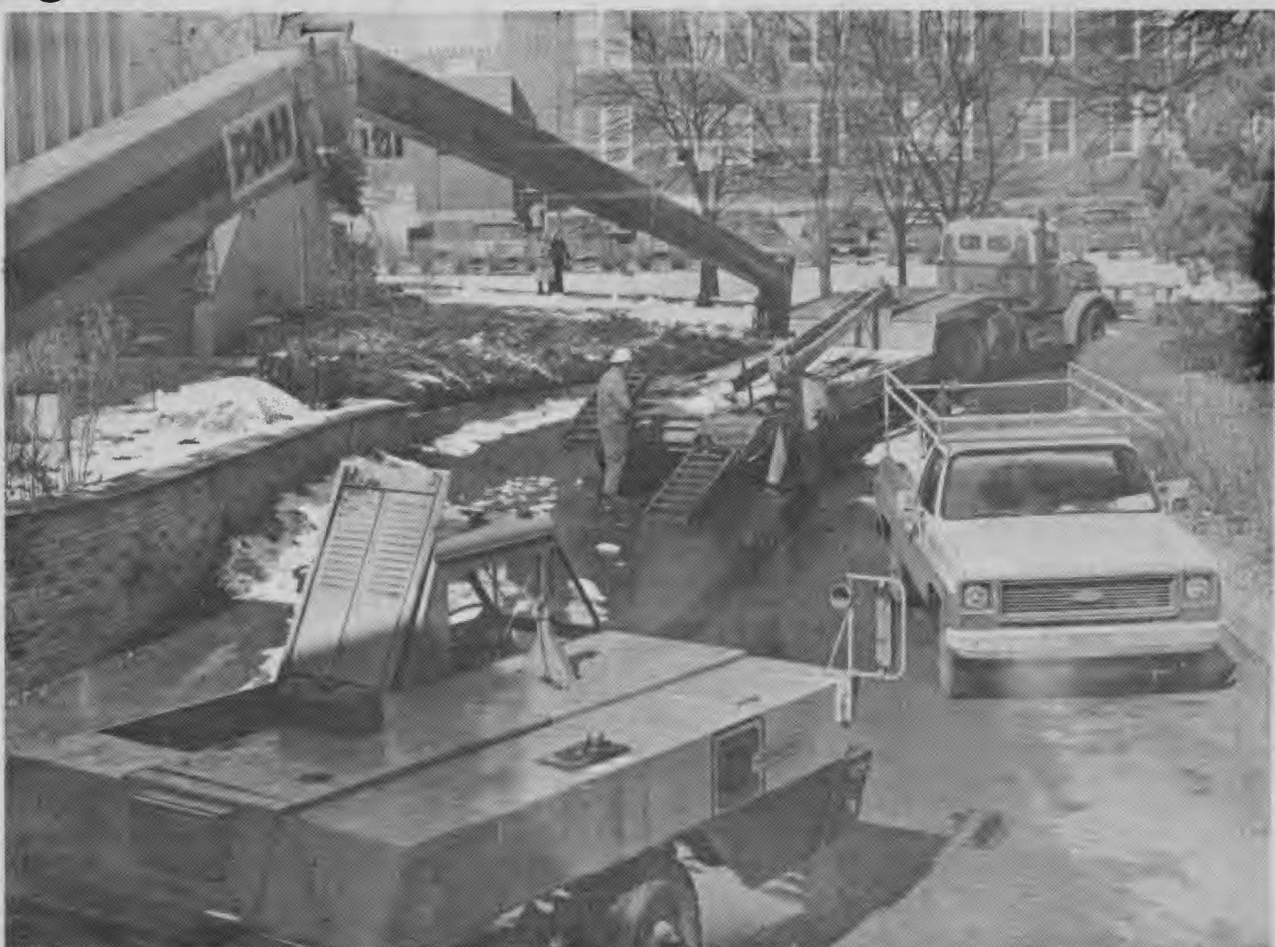
Work men examine a 30-ton crane that was damaged Tuesday in an attempt to remove a cooling tower from the roof of the University Union. Everett Alms, physical plant superintendent,
