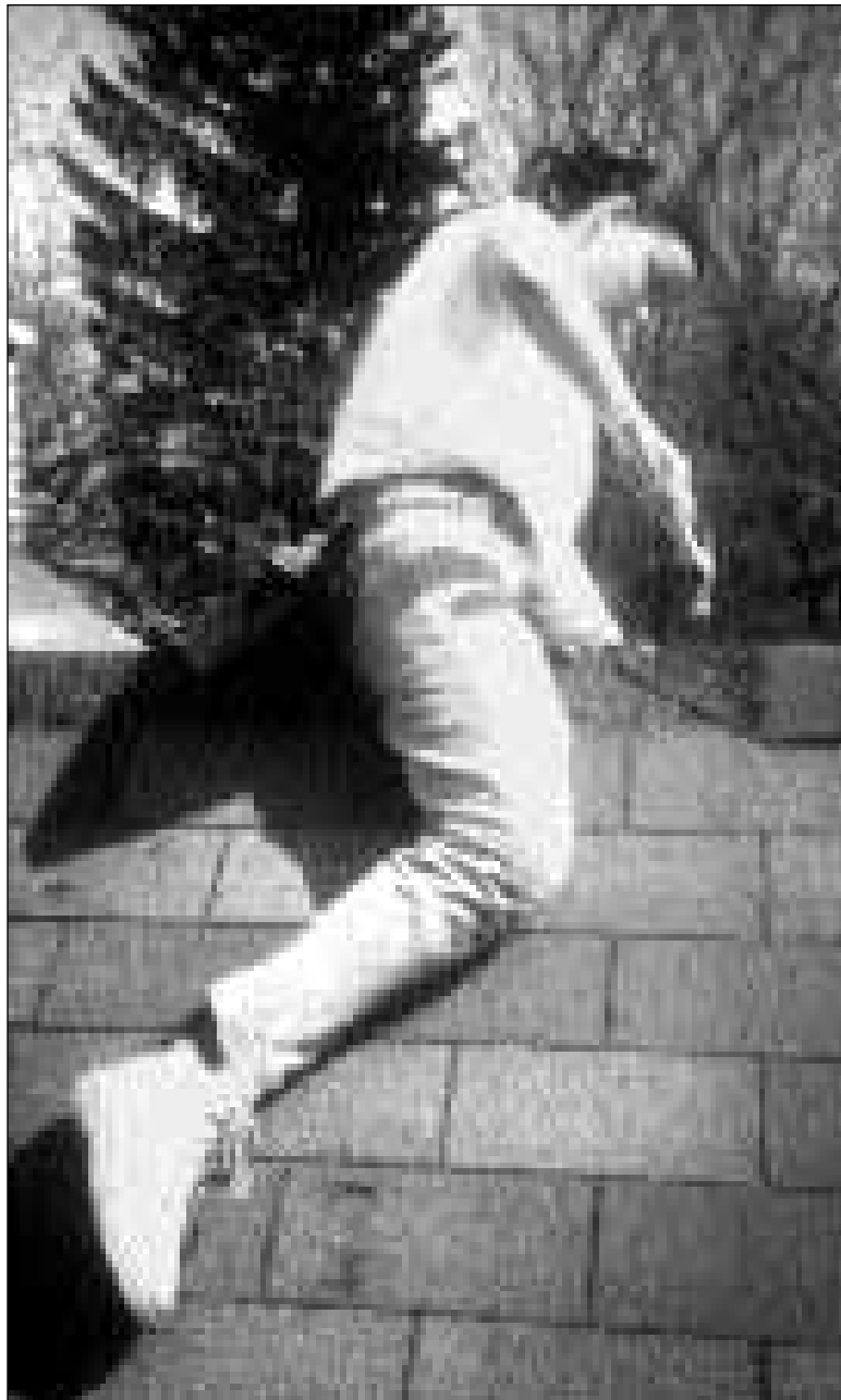
Photo courtesy of the Student Volunteer Center Nora Strong, a sophomore English major, works on a roofing project last spring during a Habitat for Humanity workshop in Battle Creek, Mich. Habitat for Humanity is one volunteer group involved with the Student Volunteer Center.
