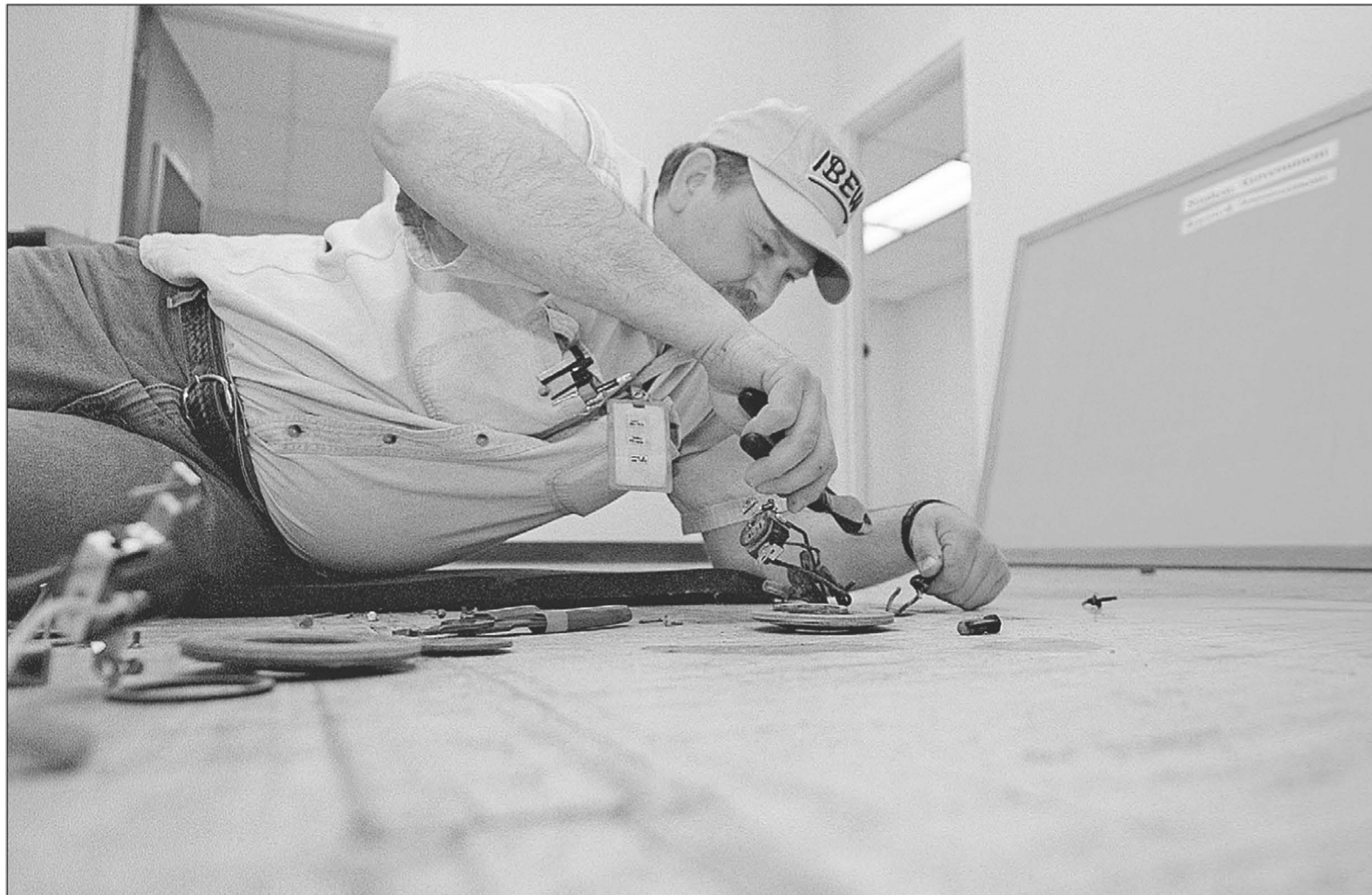
Jim Yokley of EIU electricians works on an electrical outlet in the Student Life Office Monday afternoon.
