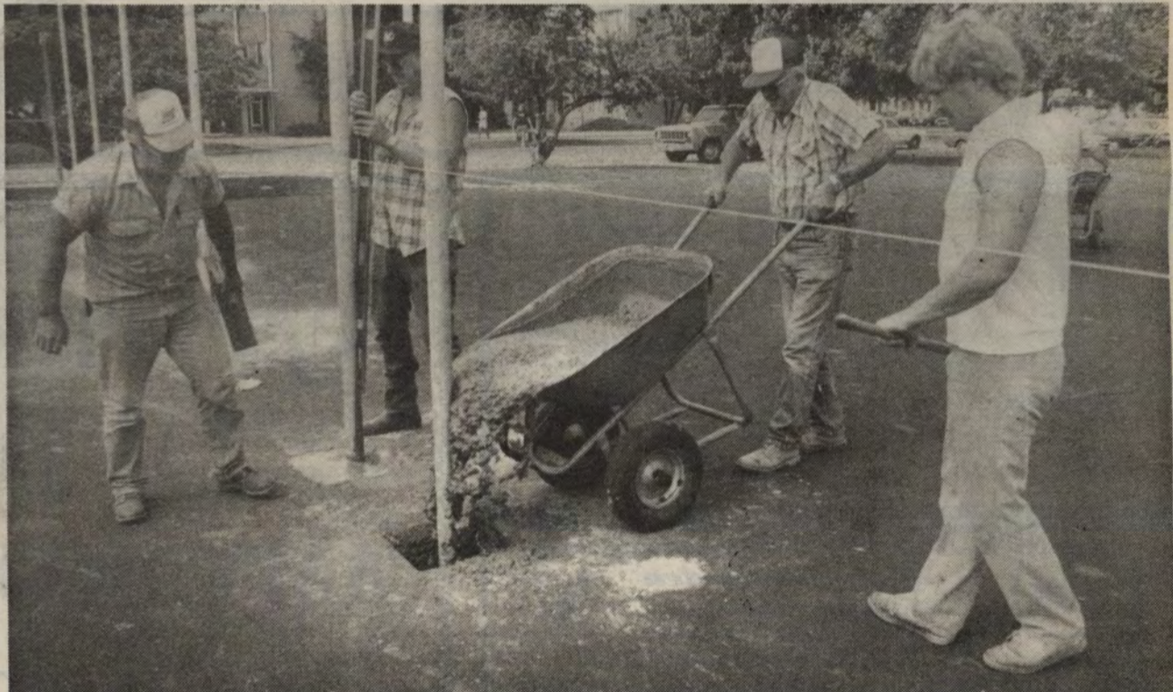
Pouring it on A quartet of Eastern groundsman pour cement for newly paved tennis courts across from Thomas Hall on Seventh Street. The four workers, from left, are Jim Dowland, Bill Griffith, Ivan Van Tassel and Jim Phillips.
