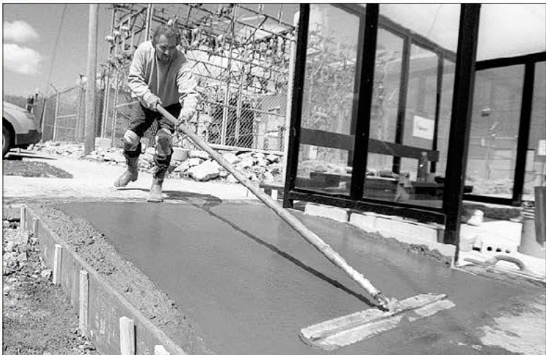
Jim Cravens, a university mason, smooths out concrete for a wheelchair ramp near the Union and the Power plant last Thursday afternoon.
