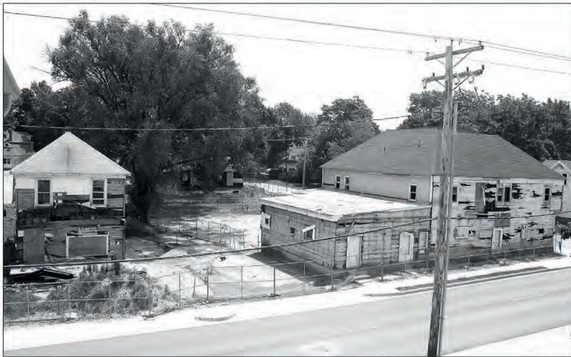
Partially demolished houses sit on the corner of Fourth Street and Polk Avenue. The houses are the subject of a lawsuit brought by the city.
