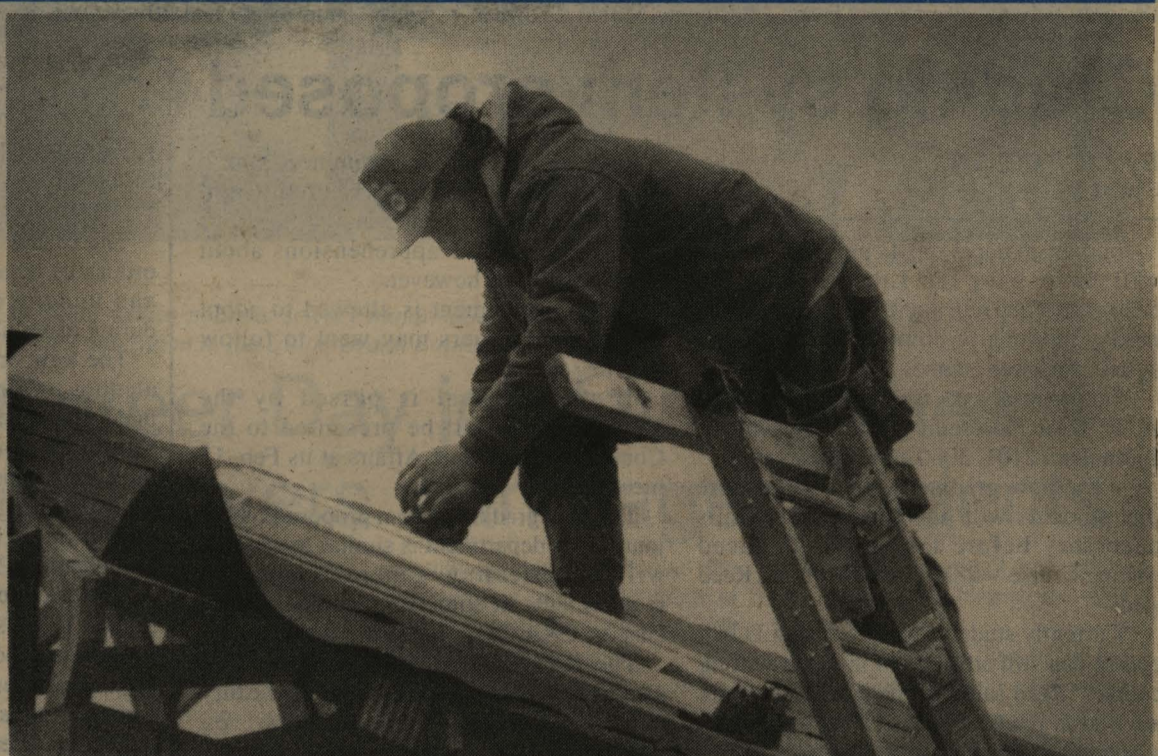
SHANNON THOMAS/Staff photographer A construction worker for Standerfer Construction Co. moves stripping for roofing tar paper on the new addition of Greek court, as construction progresses Tuesday afternoon.
