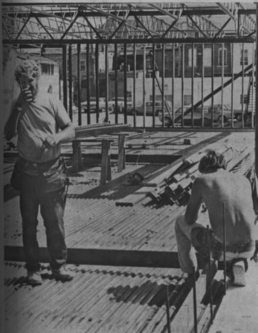
Charleston residents John Melton and Bud Easter work on construction at the First Christian Church. Frank Clinton of the Charleston Chamber of Commerce said employment is offset by the student population. (News photo by Paul Palsang)
