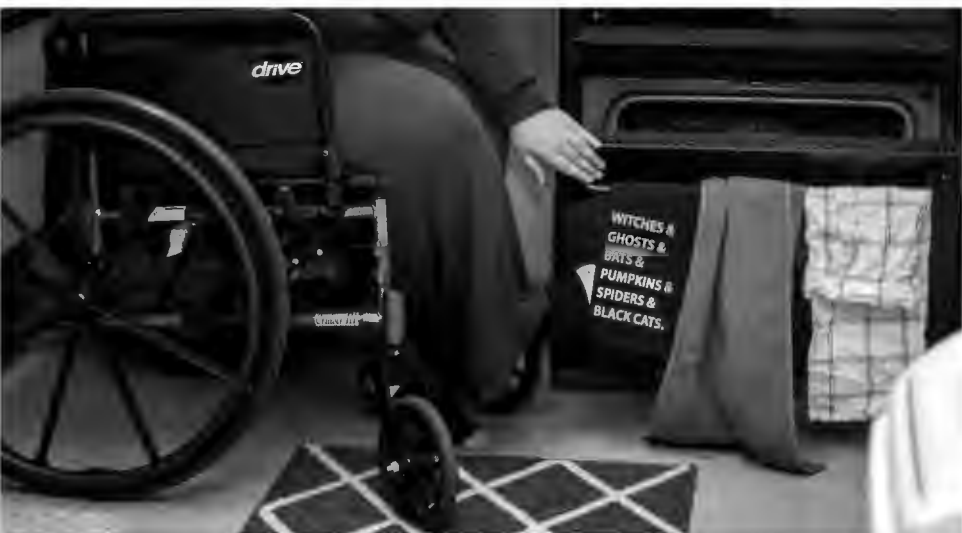
TOP: Richardson has a bathroom with two grip railings attached behind and next to the toilet. While the railing next to the toilet has all of its screws fastened into the wall, the railing behind is missing two of three screws in one of the anchor points. Richardson said they are lucky because they don't need to use the behind railing, but it upsets them because what if they, or someone else, had to?
