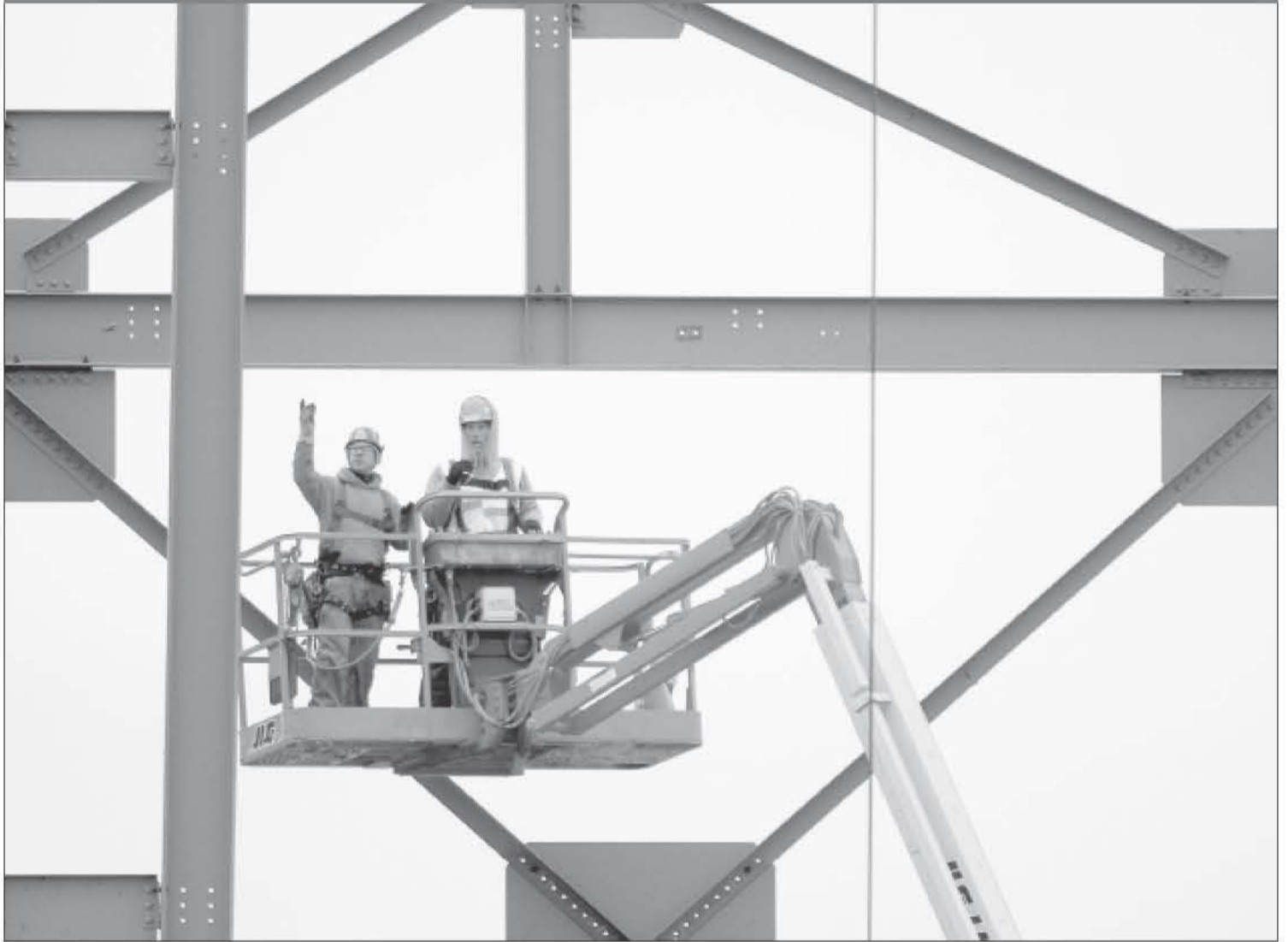
Construction workers for Shook Construction company work on a vertical lift Tuesday at the site of the Renewable Energy Center at 18th Street.
