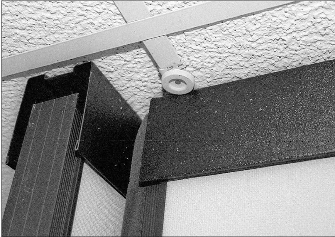
Renovations in the Student Life Office will take care of problems like this wall that is not properly aligned with the ceiling.
