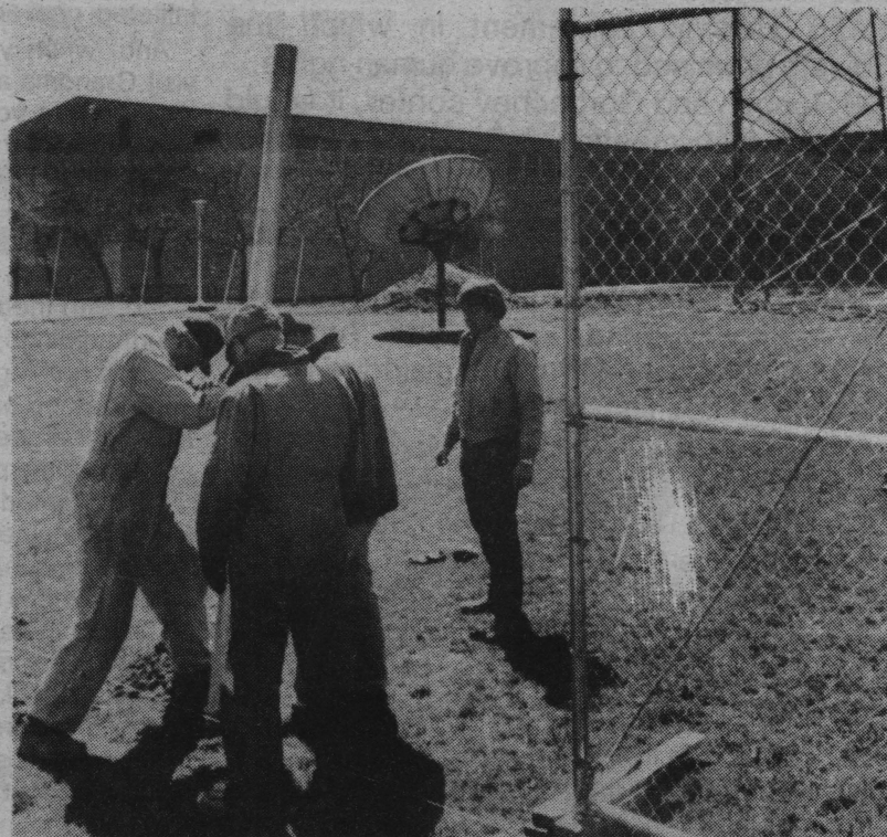
Workers install a protective fence behind Buzzard Building Tuesday as part of the Radio/TV Center's expansion. The fence surrounds a new satellite dish and antenna tower for WEIU-FM radio, a new educational radio station scheduled to go on-line July 1. (News photo by Michael Sitarz)
