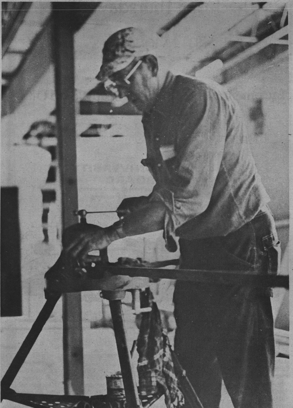
Russ Green, a pipe fitter, is threading pipe for the heaters at the textbook library. Renovation has been underway since January and is 70 percent complete. The work is scheduled to be completed by August 15. (News photo by Kenith Hathcock)
